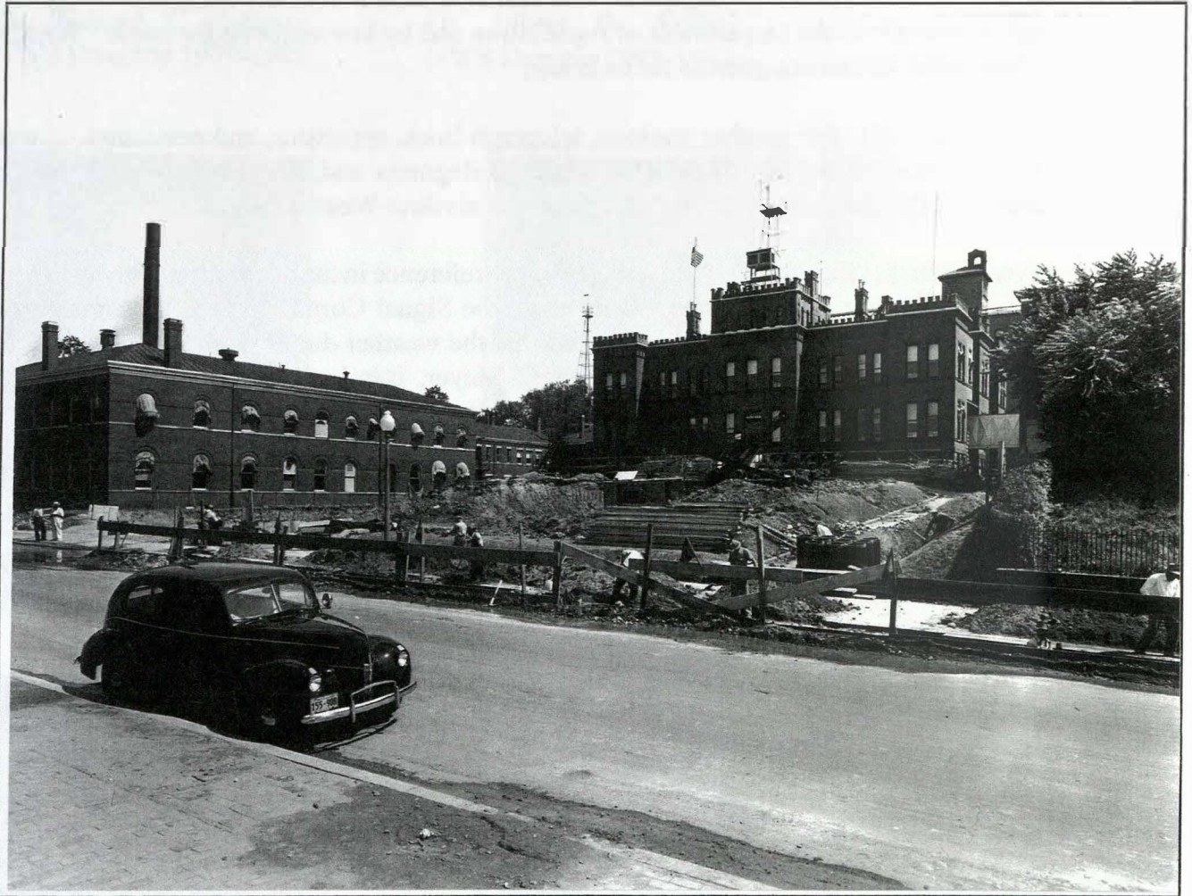
Figure 1. The Ferguson Building with the tower for measuring wind and the Old Annex to the left. The new building construction is in the foreground. Picture taken facing south-southeast.
